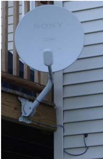
Incorrect (wires visible)
